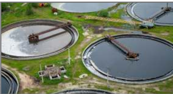
Waste water treatment plant
