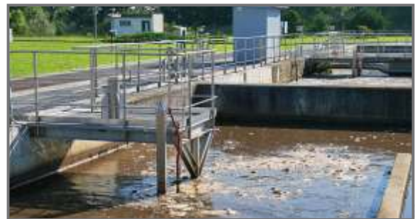
Waste water treatment plant
